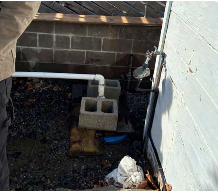
Private property sump pump system
