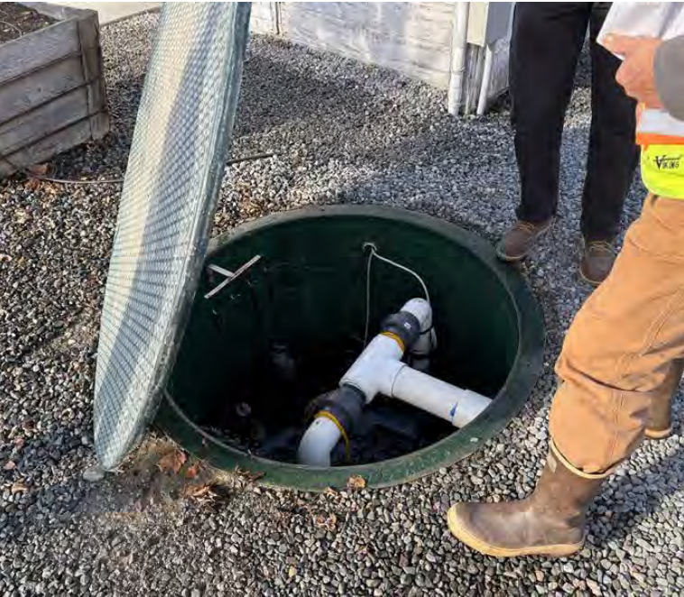
Private property sump pump system
