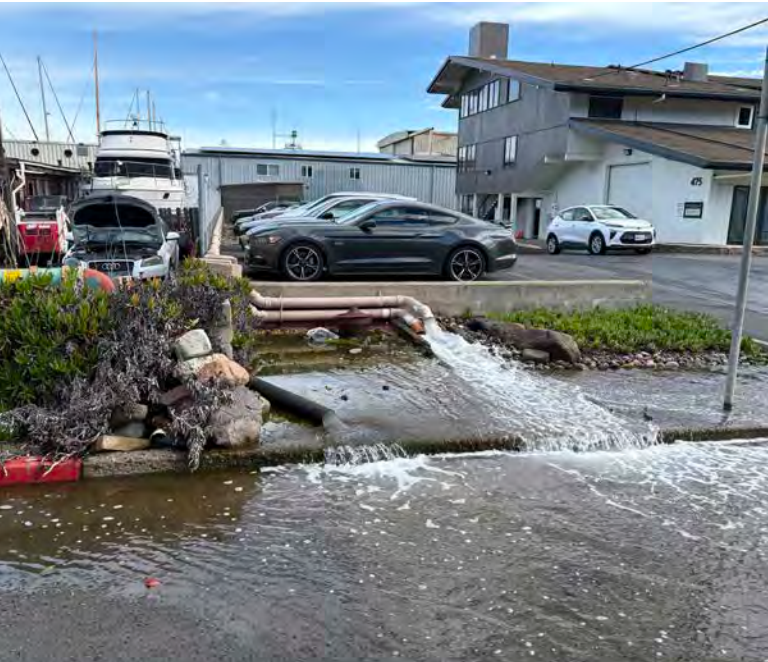
Private property pumps discharge onto Gate 5 Road
